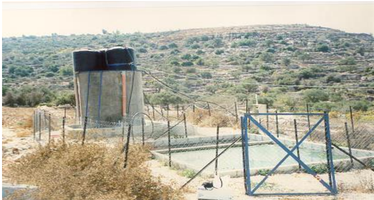
Biet-Diko wastewater treatment plant
